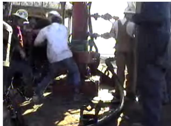
Rig crew secures casing head for vital cement job on an Enermax well in Texas.
